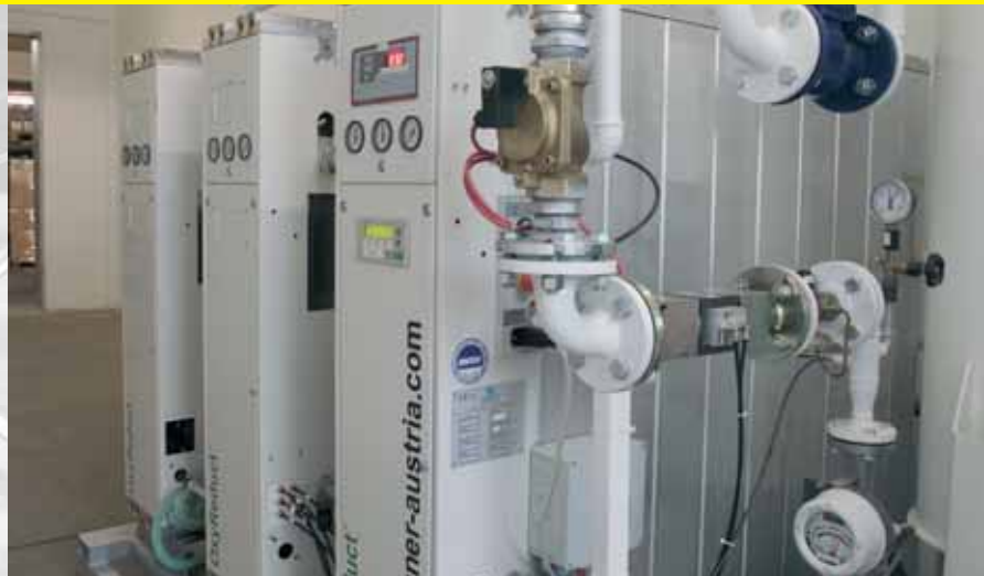
Oxy Reduct system for fire prevention
